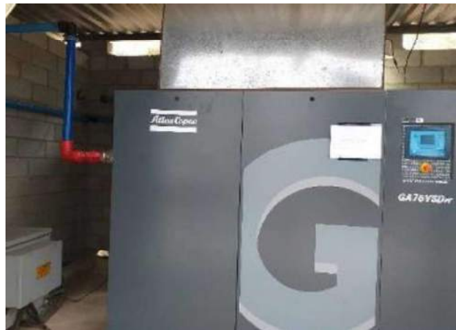
Compressor Atlas Copco
